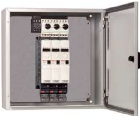
Example of GV2/Altivar 32 direct mounting in an enclosure: GV2 P self-protected disconnect + GV2GH7 line spacer + ATV 32HU15N4 drives
